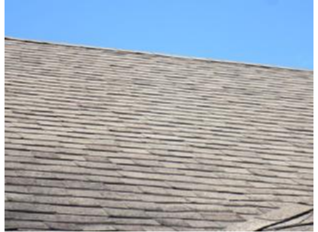
The roof shows damaged shingles, and some loss of mineral granules. Recommend that entire roof be evaluated by
