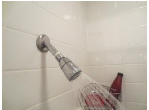
Shower head was leaking as seen in photo 6.
