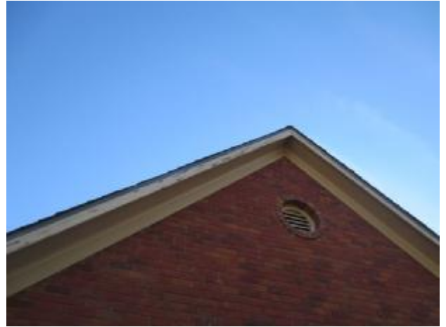
Wood trim showed signs of paint peeling, loose caulking, delamination, moisture penetration in several areas,
