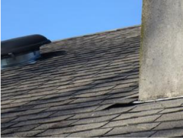
The roof shows damaged shingles, and some loss of mineral granules. Recommend that entire roof be evaluated by
