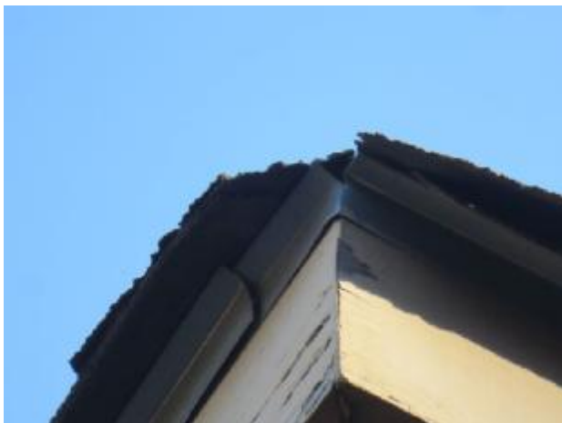
The roof shows damaged shingles, and some loss of mineral granules. Recommend that entire roof be evaluated by
