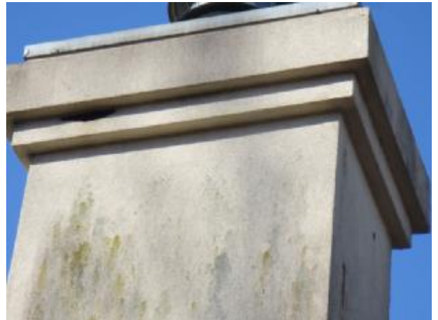
Exterior Insulated Finish System (EIFS) has been known to be susceptible to water problems which can cause serious structural damage. Full EIFS inspection requires penetration of
