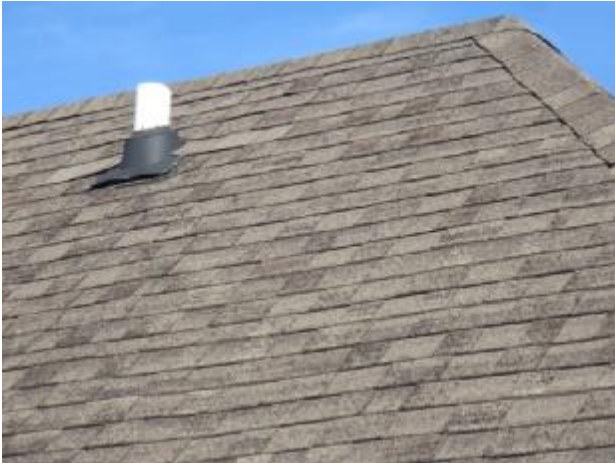
The roof shows damaged shingles, and some loss of mineral granules. Recommend that entire roof be evaluated by
