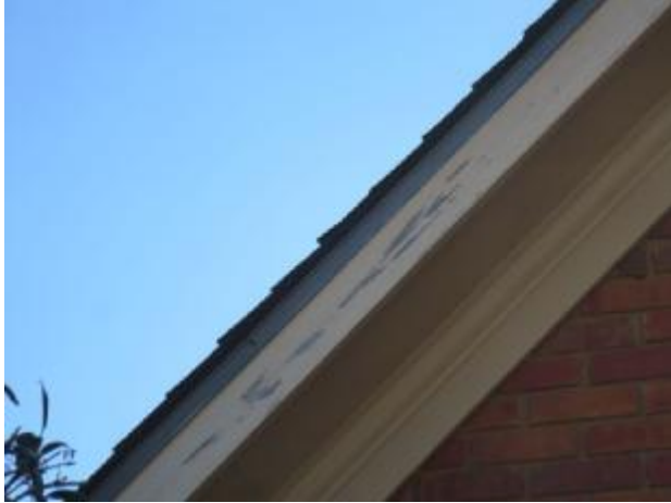
Wood trim showed signs of paint peeling, loose caulking, delamination, moisture penetration in several areas,
