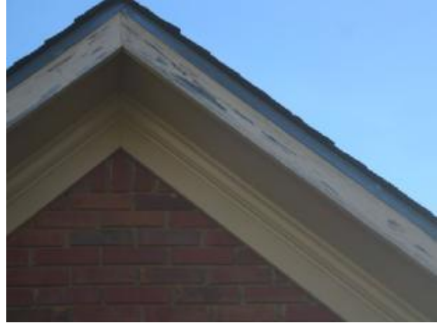
Wood trim showed signs of paint peeling, loose caulking, delamination, moisture penetration in several areas,
