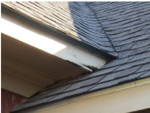
Wood trim showed signs of paint peeling, loose caulking, delamination, moisture penetration in several areas,
