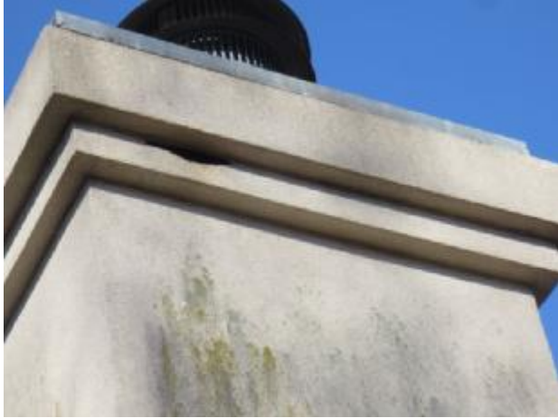
Exterior Insulated Finish System (EIFS) has been known to be susceptible to water problems which can cause serious structural damage. Full EIFS inspection requires penetration of
