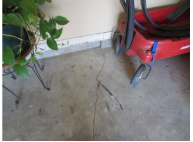
Some cracks were present in garage as seen in foundation photos where cracks are visible. Recommend further
