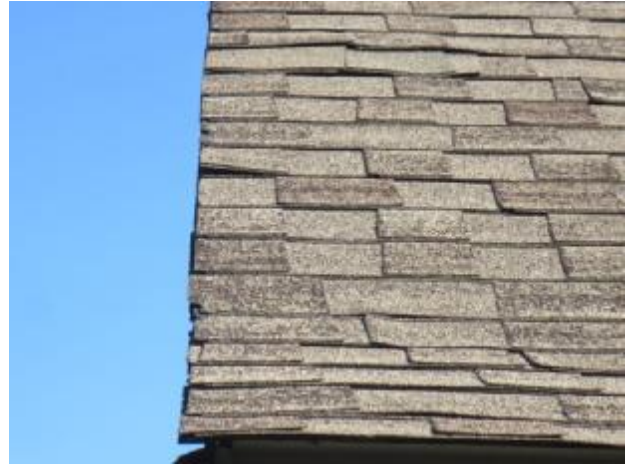
The roof shows damaged shingles, and some loss of mineral granules. Recommend that entire roof be evaluated by
