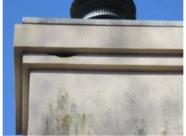
Exterior Insulated Finish System (EIFS) has been known to be susceptible to water problems which can cause serious structural damage. Full EIFS inspection requires penetration of
