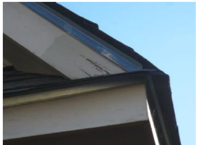
Wood trim showed signs of paint peeling, loose caulking, delamination, moisture penetration in several areas,
