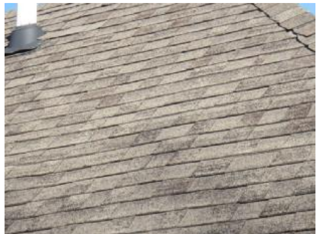
The roof shows damaged shingles, and some loss of mineral granules. Recommend that entire roof be evaluated by
