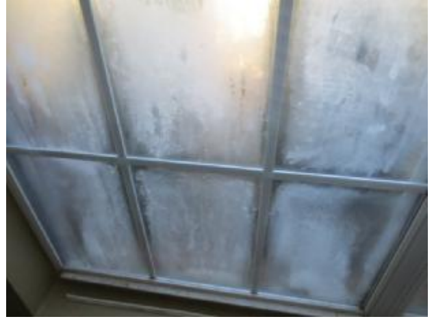
The window at front bedroom appeared to have a defective insulator panel at bottom. Recommend that a licensed building
