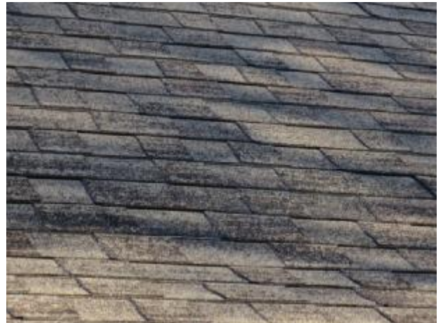
The roof shows damaged shingles, and some loss of mineral granules. Recommend that entire roof be evaluated by
