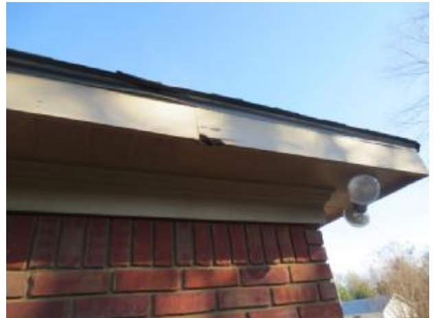
Wood trim showed signs of paint peeling, loose caulking, delamination, moisture penetration in several areas,
