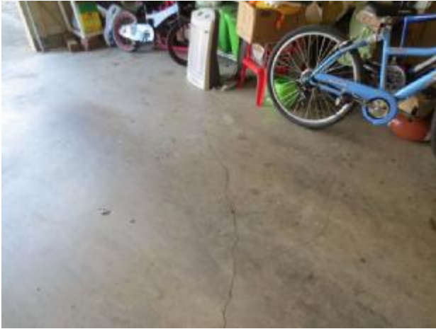
Some cracks were present in garage as seen in foundation photos where cracks are visible. Recommend further
