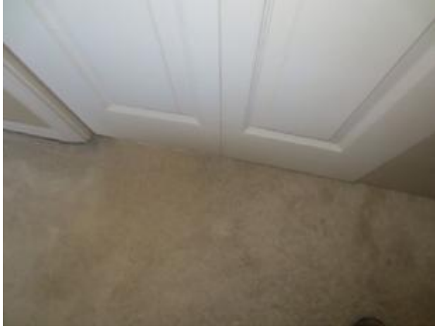
Closet door at front bedroom closet needs adjusting at bottom right. (see photo 12 and 13).
