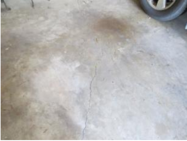
Some cracks were present in garage as seen in foundation photos where cracks are visible. Recommend further
