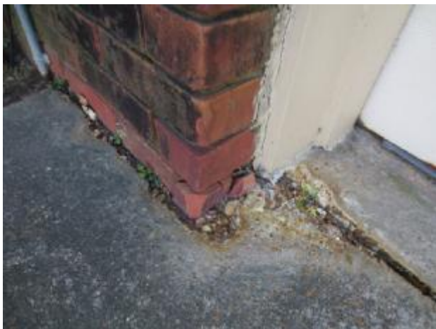
Wood trim showed signs of paint peeling, loose caulking, delamination, moisture penetration in several areas,
