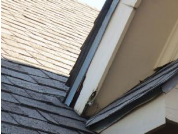
Wood trim showed signs of paint peeling, loose caulking, delamination, moisture penetration in several areas,
