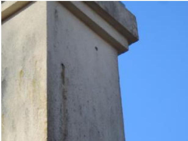
Exterior Insulated Finish System (EIFS) has been known to be susceptible to water problems which can cause serious structural damage. Full EIFS inspection requires penetration of
