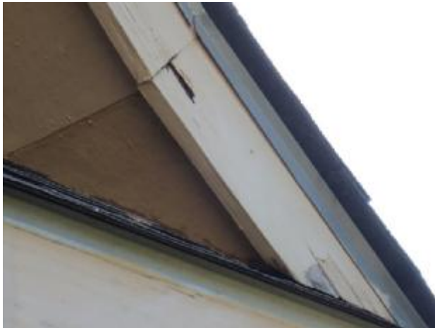
Wood trim showed signs of paint peeling, loose caulking, delamination, moisture penetration in several areas,
