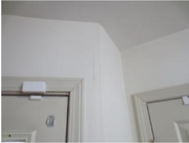
Some areas in home at walls and ceiling need repair and paint. (Closet in master bath. Also see ceiling photo at master bedroom for interior room photo) (see photo #12 and 13)
