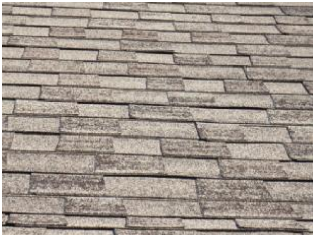
The roof shows damaged shingles, and some loss of mineral granules. Recommend that entire roof be evaluated by
